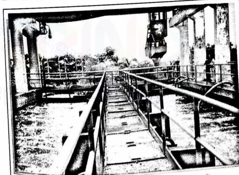
Photo Fig. 9.1 (b) Photoview of the two of the four grit channels (outfall end side) provided after the fine screens at the Ghatkopar Sewage Treatment Plant, Mumbai.
