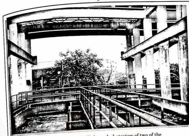
Photo Fig. 9.1 (a) Enlarged photoview of two of the four grit channels (entry side) provided after the fine screens at the Ghatkopar Sewage Treatment Plant, Mumbai.
